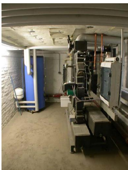
Figure 3: left hot water tank, right district heating connection station (Source: Parabel Energiesysteme GmbH)
