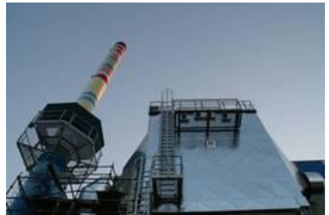
Figure 8: Biomass power plant (Source: KPG)
