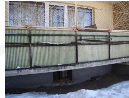
Pic.12, Loggia of a 12-floor multi-apartment building in Jugla [3]
