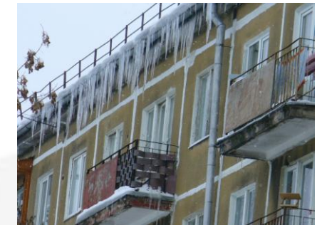
Pic.13, intensive heat losses (a multi-apartment building in Jugla). [3]
